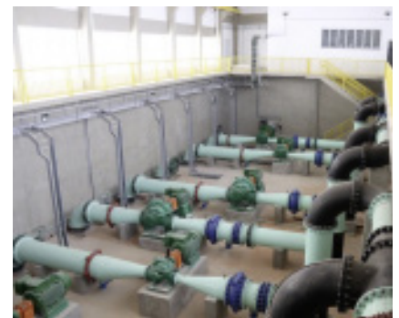
VCW fast check valves installed on the water line.
